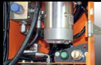
Oil fill pump
