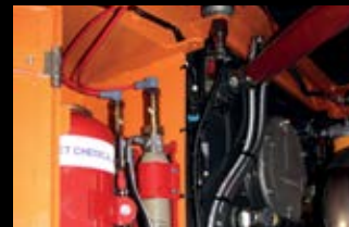
Fire suppression system
